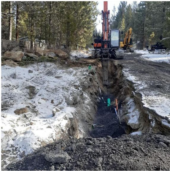
Figure 2: Image of the jack-hammering completed along the North Main St line, not the piles of removed broken bedrock on the left of the picture. This will be removed once work is completed and clean-up operations occur.
