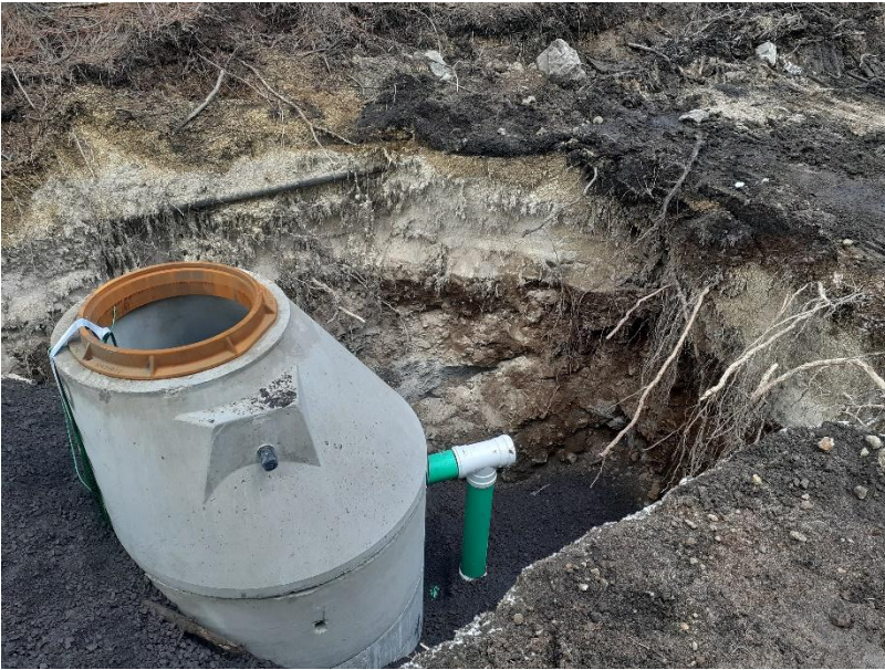
Figure 2: Image of the dropped manhole completed along the North Main St line.
