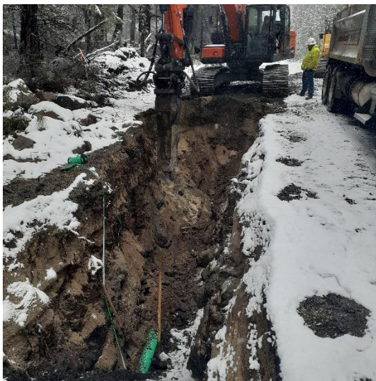
Figure 1: Image of a mainline trenchwork and jack-hammering along the north Main St crew.
