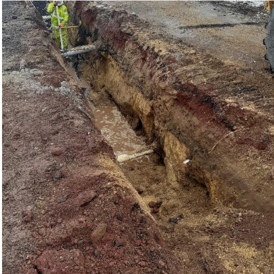
Figure 2: Image of mainline being laid on south Main St crew. Note the many utility conduits shown in the picture. Half of what is shown were unmarked.
