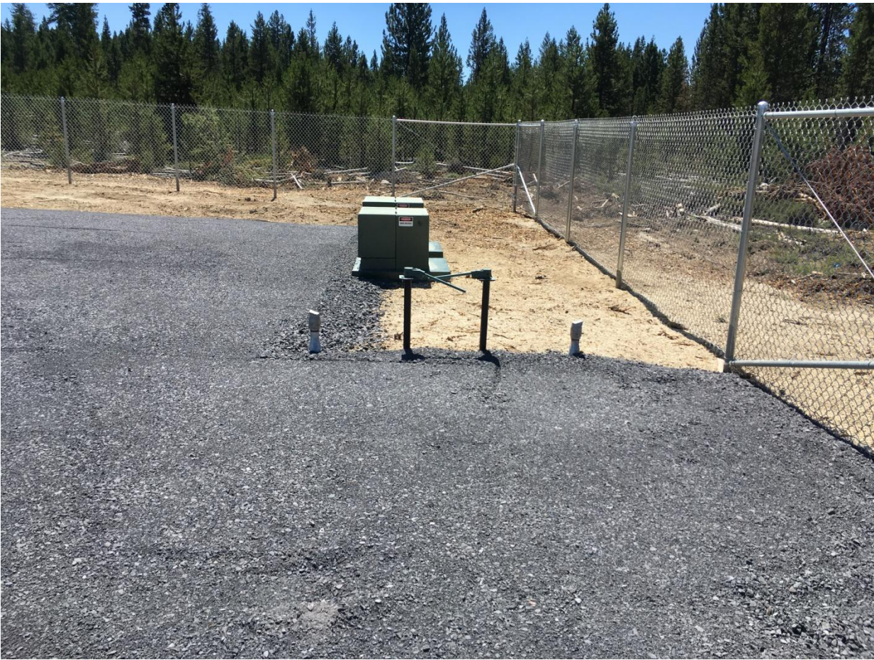
Figure 1: Looking south at the irrigation fields on/off valves to direct recycled waters to either irrigation field if needed in the future.
