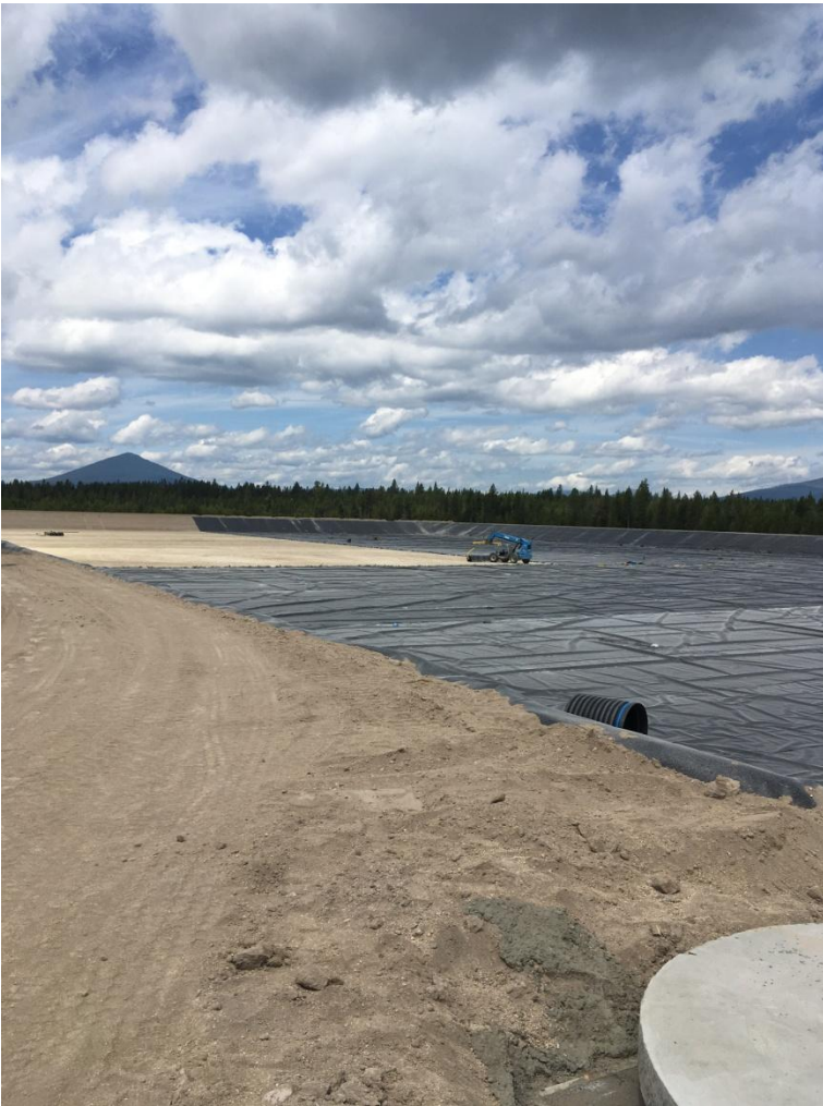
Figure 7: Looking west at liner operations in the storage pond. Only the southwest leg of the pond remains to be completed.
