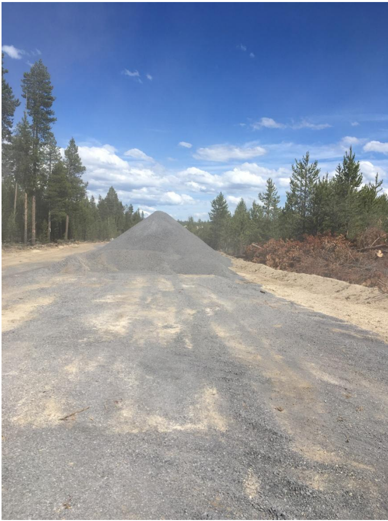
Figure 6: Looking east at the graveled access road that leads from the pipeline crossing to the NW corner of the facility. Note the gravel mound on hand that will be spread to create the remainder of the gravel roads in the facility.
