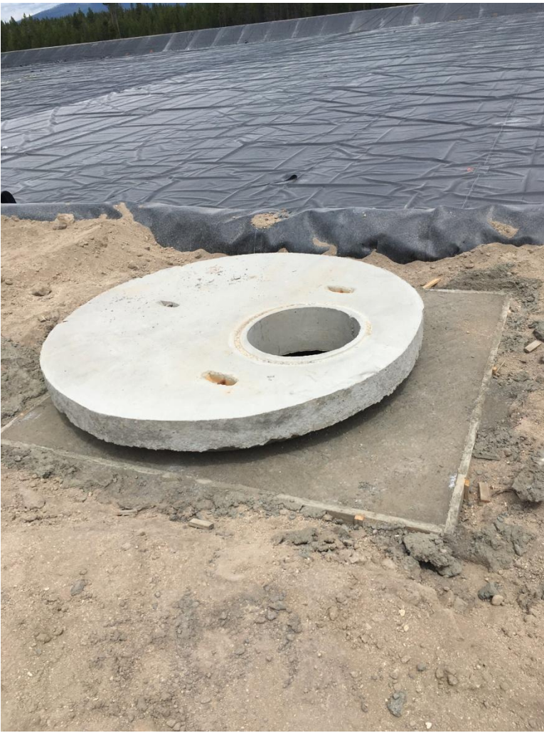
Figure 3: Riser lids have been placed with surrounding rat slab for support along the chlorinator.
