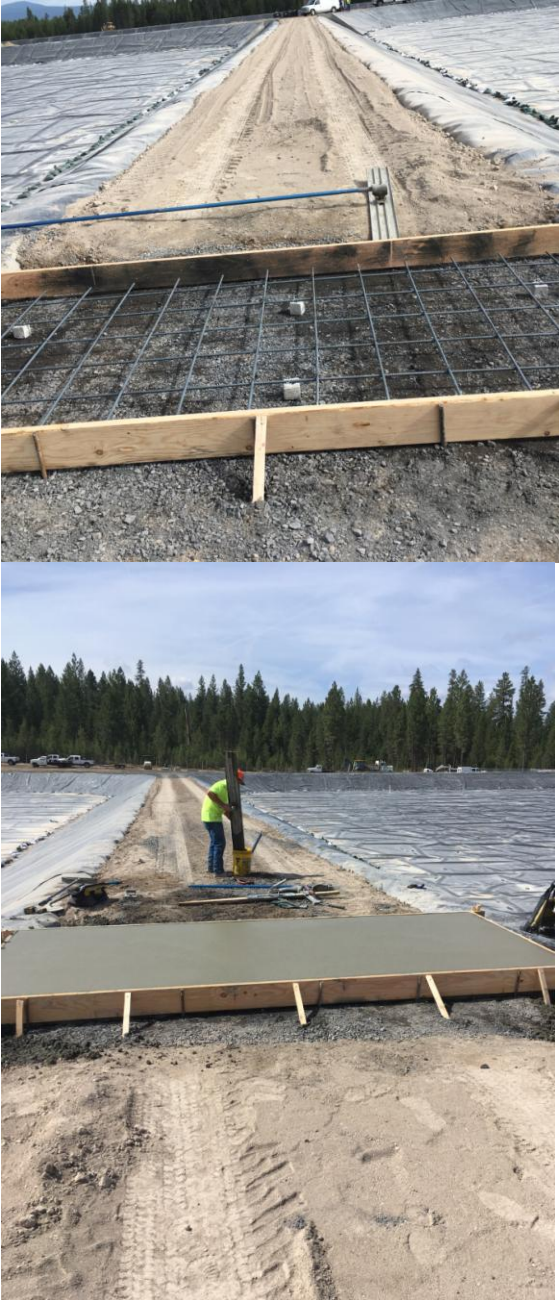
Figure 1: A before and after picture of the walkway atop the crossflow structure between the two lagoons. Note the correct spacing and placement of rebar.
