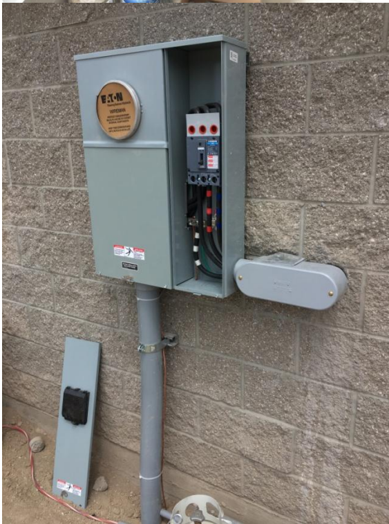
Figure 2: Looking inside and outside the chlorination building at the junction boxes ready for power hookups by mid next week.
