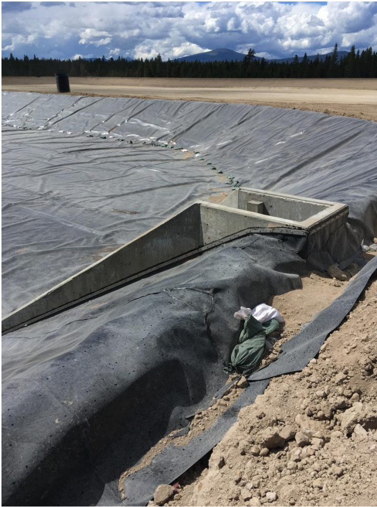
Figure 5: Looking northwest at the western lagoon that is lined. Note that the liner is bolted to the crossflow structure walls to ensure a complete seal.
