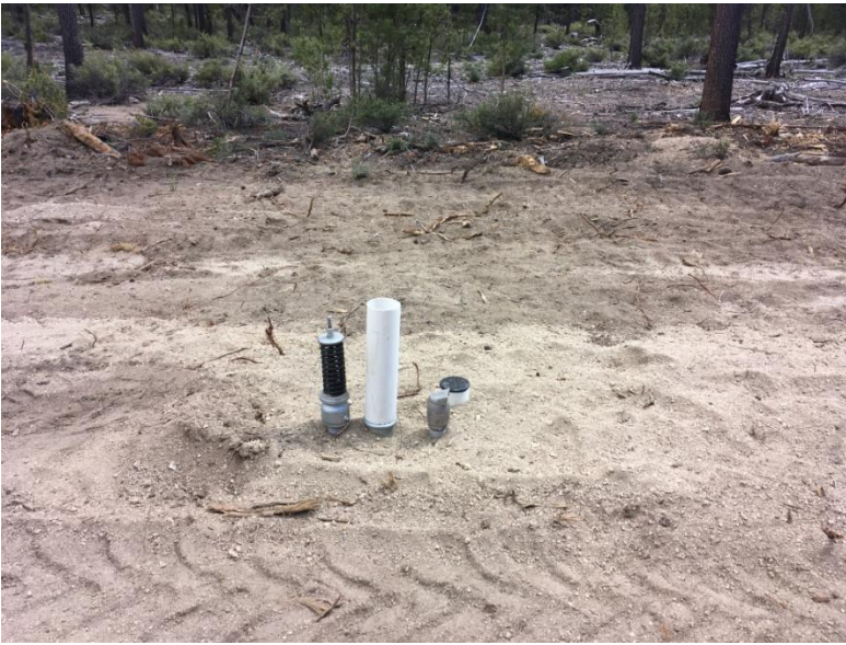
Figure 3: Looking south at the stub out of the irrigation mainline. Note the clean out.
