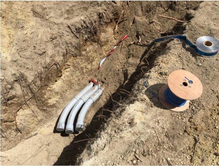
Figure 1: Trench with the electrical conduits waiting for connection. This image is on the east side of the gasline crossing.
