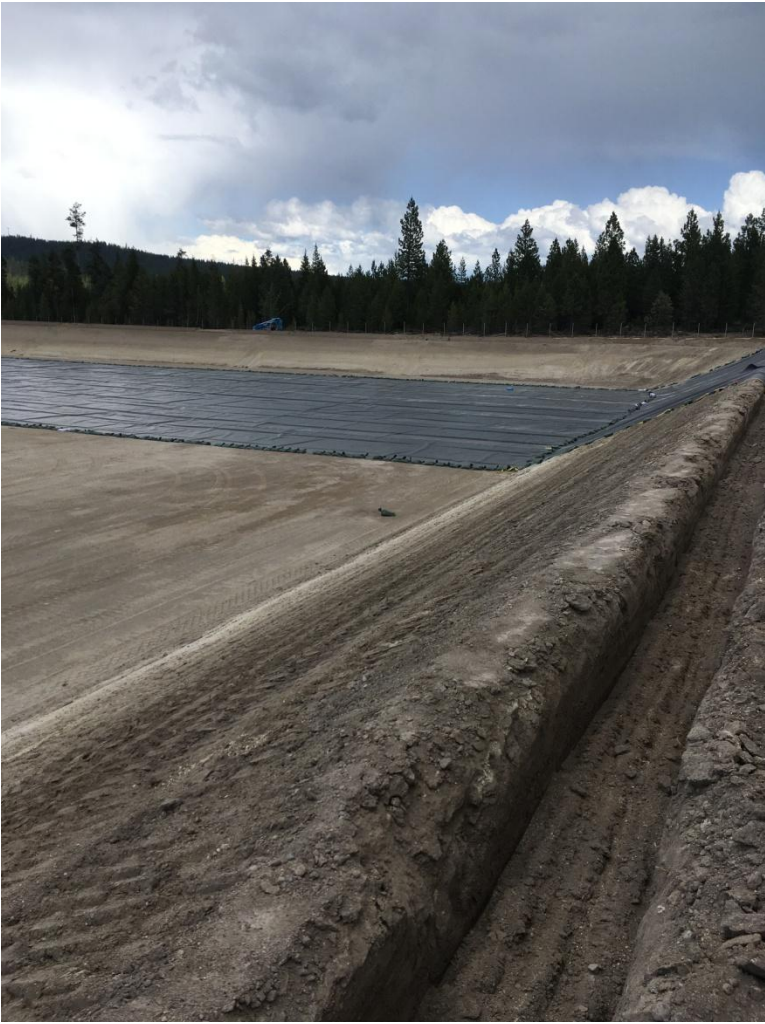
Figure 8: Looking east at the start of lining operations for the storage pond.
