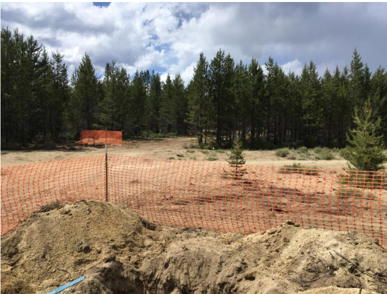
Figure 2: Looking west from the east side of the gasline crossing trench, to the mirrored trench on the west.
