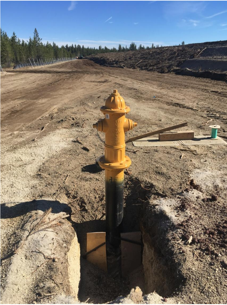
Figure 5: The installed fire hydrant to be used for dust suppression by the fire service.
