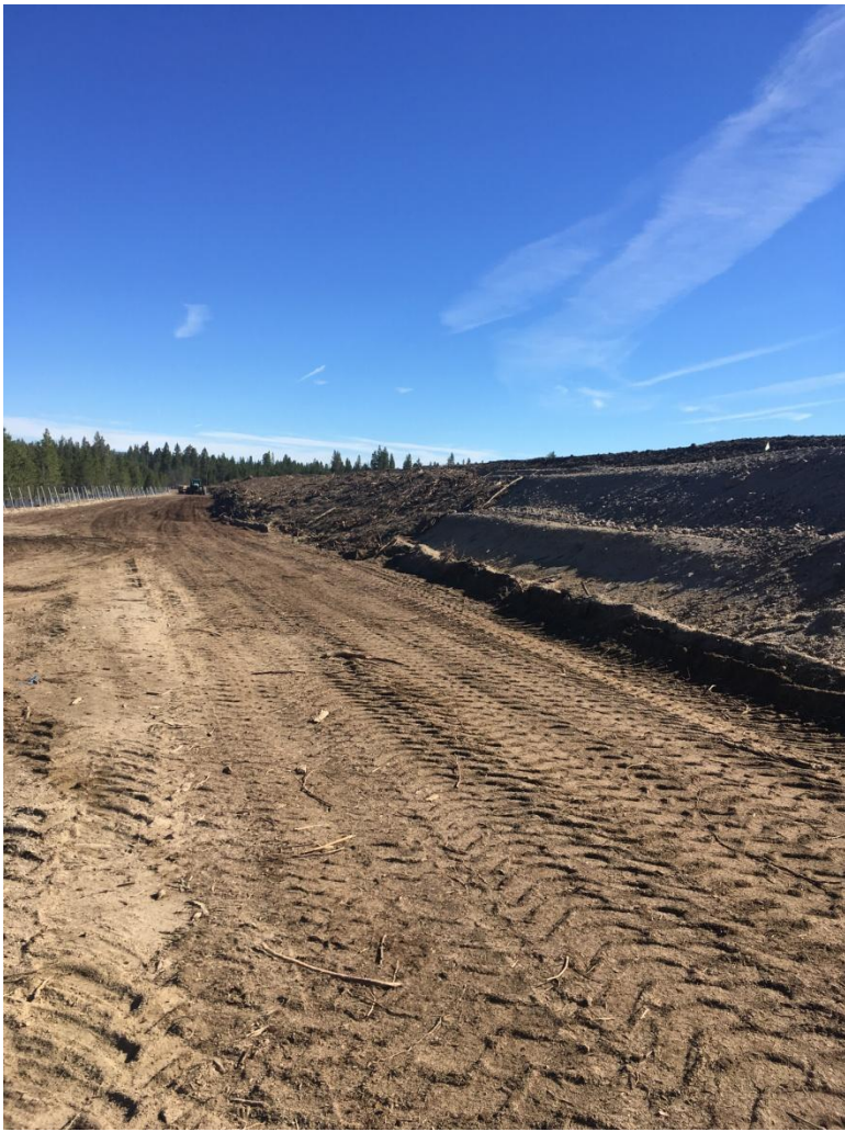
Figure 4: Looking north at the western-most berm along the storage pond. Note that amouring has been completed on the northern slope, to about half way through the picture with material stacked and waiting for amouring to be complete.
