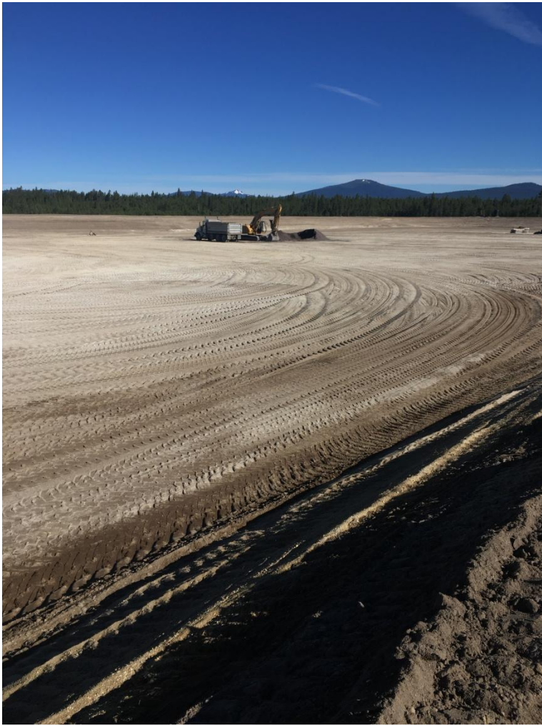
Figure 2: Looking north at the western lagoon. Note the lagoon is to grade, minus the small amount of staging materials that will be removed before liner operations begins in this lagoon.
