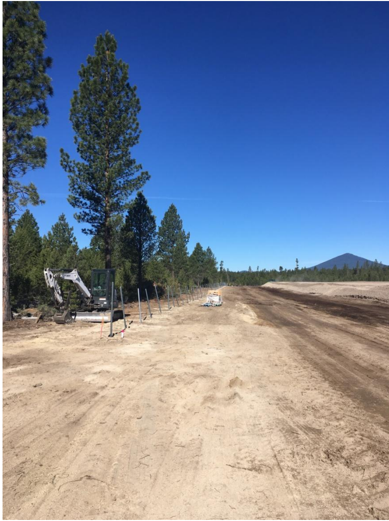
Figure 3: Looking west at the placement of fence poles for the cyclone fence that will run the perimeter of the facility.
