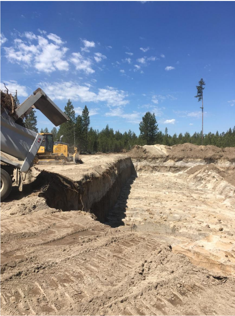
Figure 2: Looking west at a large trench dug to place displaced tree and root materials that are not needed while clearing the irrigation main line access road.
