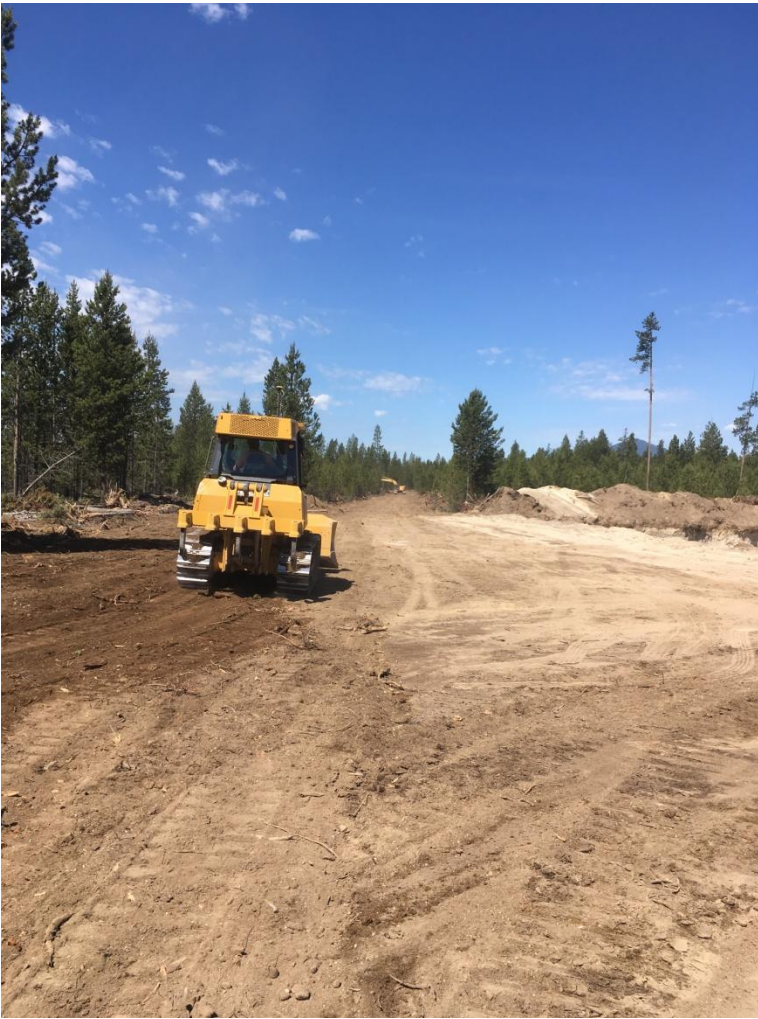
Figure 1: Looking west at the irrigation main line being cleared in order to lay pipe and eventually create an access road.
