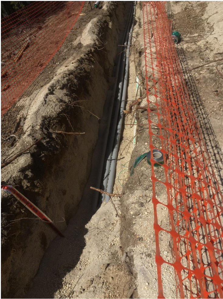
Figure 3: Looking west at the electrical conduits in place and awaiting connection to the grid after the gasoline crossing is completed.
