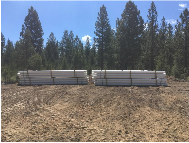
Figure 6: Irrigation lines on hand and awaiting installation. These white pipes will be marked by a purple strip to specific non-potable, reclaimed water, as per DEQ regulations.
