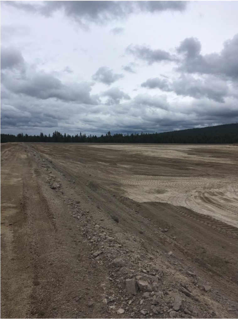
Figure 1: Looking north while driving on the storage pond berm. The berm is 4' short from the planned elevation. Note the smooth and consistent grade of the bottom of the storage pond.
