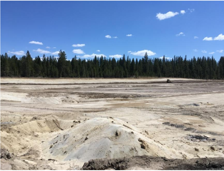
Figure 3: Looking east at large-scale discing operations. Materials are being removed from the appropriate stratigraphic layer to be mixed with pumice sands and gravels.
