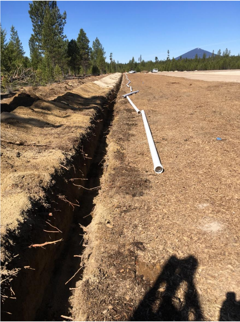
Figure 4: Looking west at the trench that they will lay the sewer line in.
