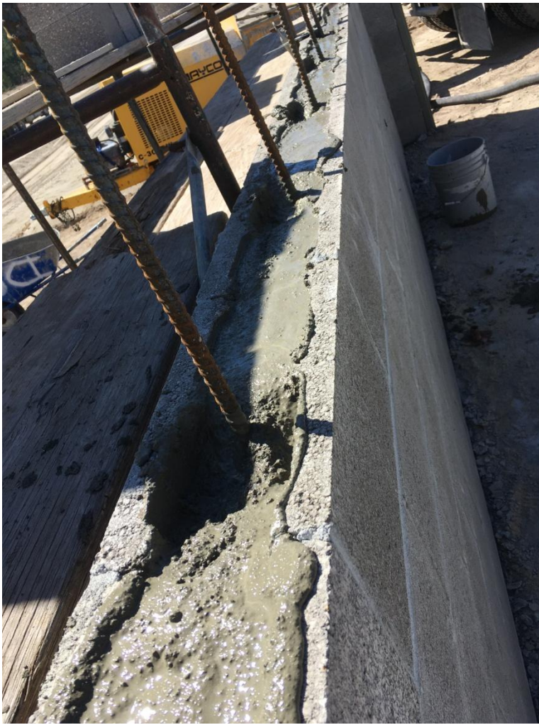
Figure 6: Concrete operations to fill in the chlorination building walls. Note that the rebar was position to stand vertically and in the center of the precast concrete blocks.
