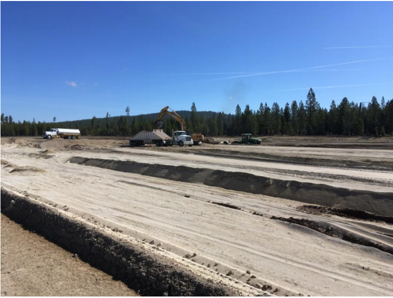
Figure 1: Looking northeast at the excavator moving materials into the belly dump for discing operations.
