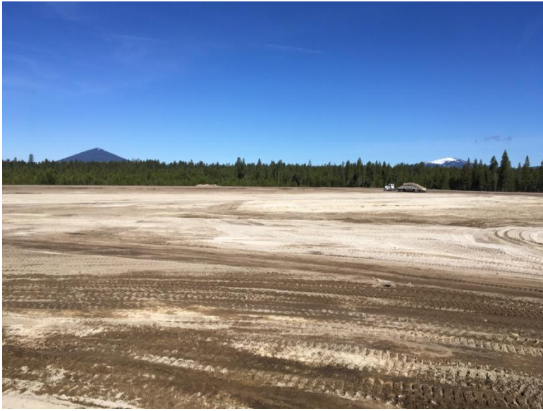
Figure 3: Looking northwest at the nearly completed storage pond. Note the belly dump in the background delivering dirt for discing operations.
