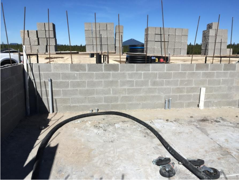
Figure 2: Looking west at the interior of the chlorinator building. Note the pipes and conduits awaiting connection.
