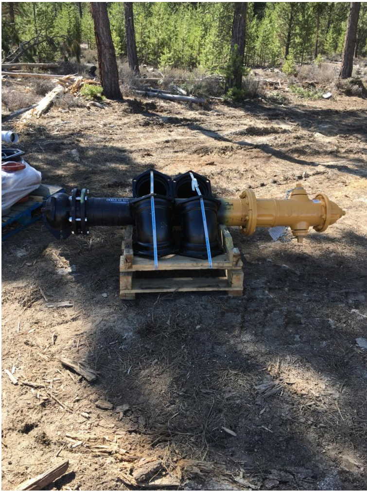
Figure 5: Materials on site – the fire hydrant.
