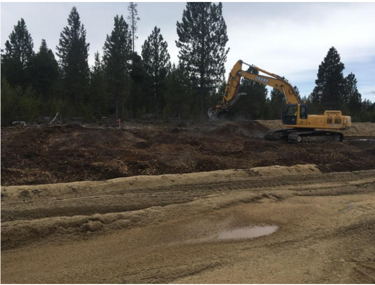
Figure 1: Looking south at the dirt being moved to make space to lay sewer lines and electrical conduits.
