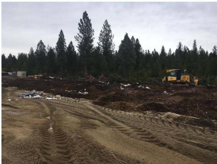
Figure 2: Looking southeast at dirt being moved to make space to lay sewer lines and electrical conduits.
