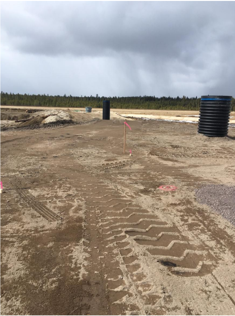
Figure 2: Looking west at the new soil blend used to build up the berm. Note the lack of tire treads. Note the risers in the background and the lift station in the far back center of the picture.
