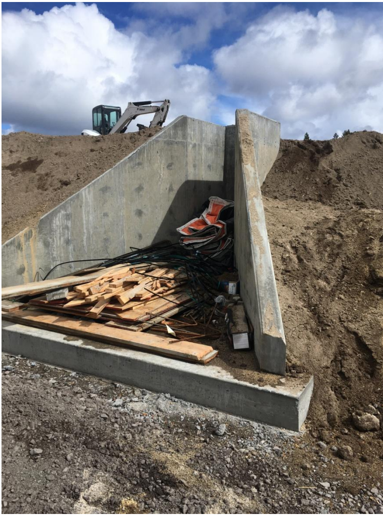
Figure 5: Looking east at the slab and walls recently poured for the crossflow structure.
