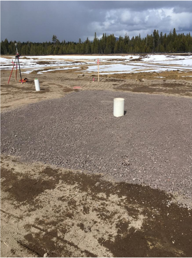
Figure 1: Looking north at the rocky pad where the chlorination building will sit. Notice the two pipe opening set up and awaiting connection to the system.
