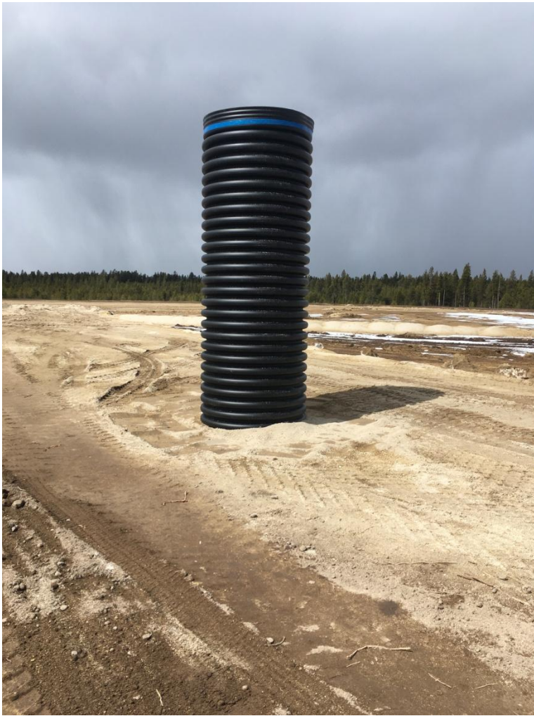
Figure 3: Looking northwest at one of the risers seated on the chlorinator.
