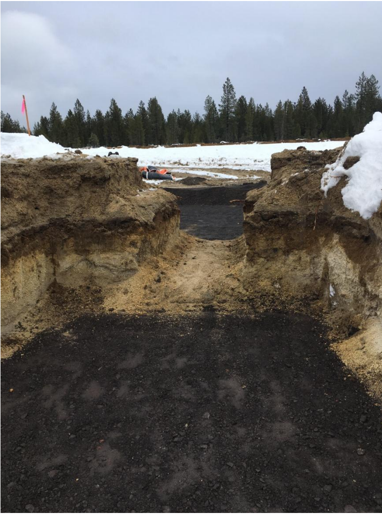
Figure 1: Looking east at the excavated pre-staked wing wall crossflow structure. Note the compressed rock at the base of the trench to provide support to the overall structure.
