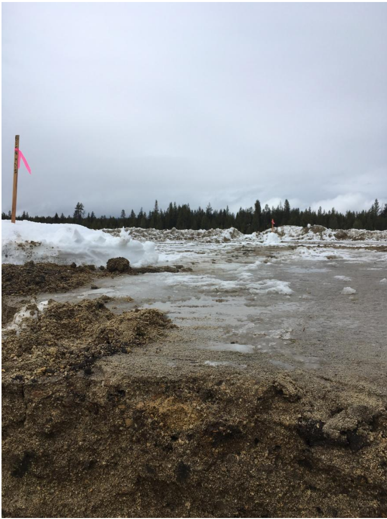
Figure 2: Looking northwest from within the trench see in Figure 1. This is the future location of the Chlorinator.
