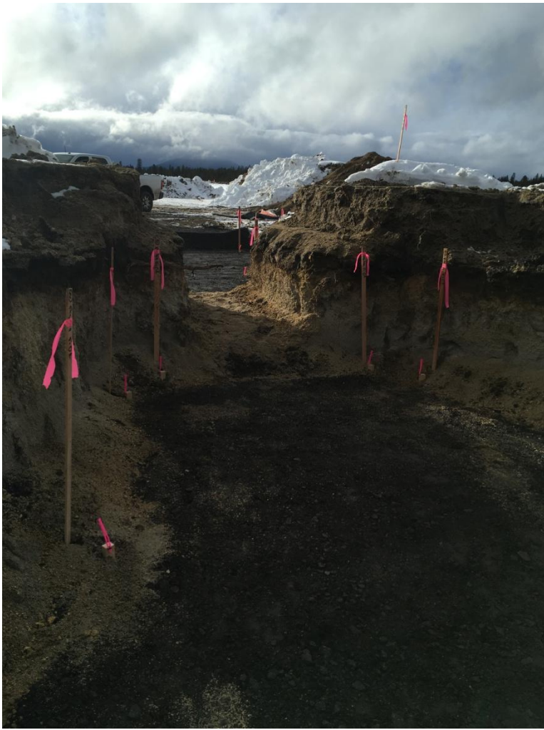
Figure 3: Looking west at the staking completed to support the construction of the wing wall crossflow structure.
