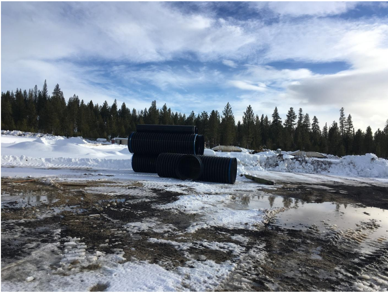
Figure 4: Looking south at the chlorinator pipe being staged on the ground prior to installation.
