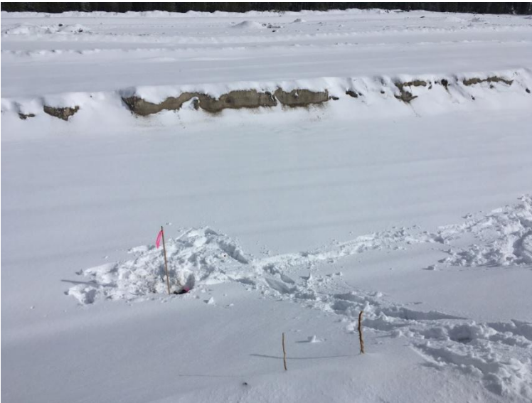
Figure 6: Looking east at staking performed to install the crossflow structure between the lagoons.
