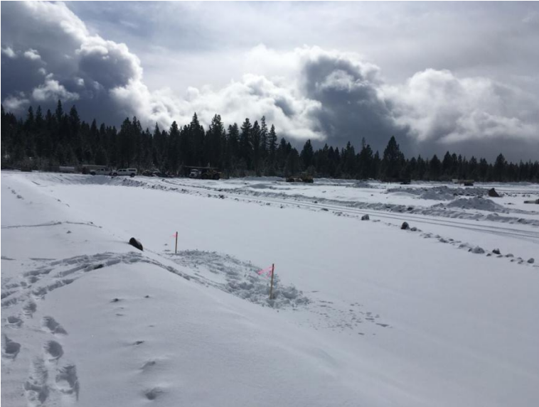
Figure 4: Looking southwest at staking done to mark a NS line of one edge of the crossflow structure between the lagoons.
