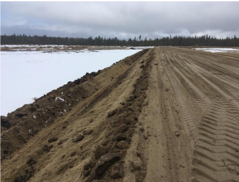
Figure 2: Looking north at the berm between the western lagoon and the storage pond. This area has been compacted to over 90%. Note the tire marks and slump forming at the sides of the berm.
