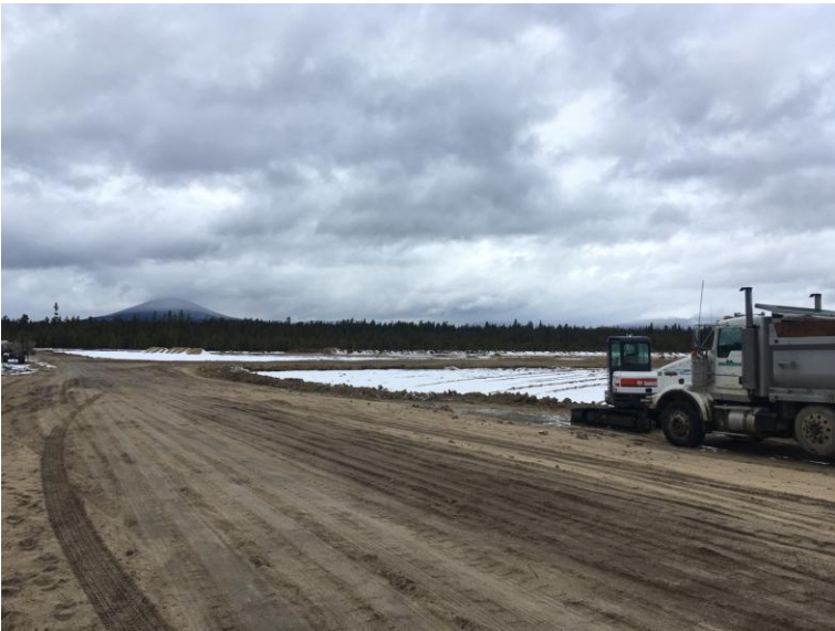
Figure 6: Looking west at the corner of the western lagoon, with the separation berm and storage pond in the background.
