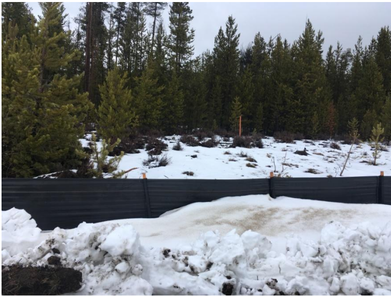
Figure 3: Looking north at the silt fence. Silt fence is approximately 47' south of the property boundary.
