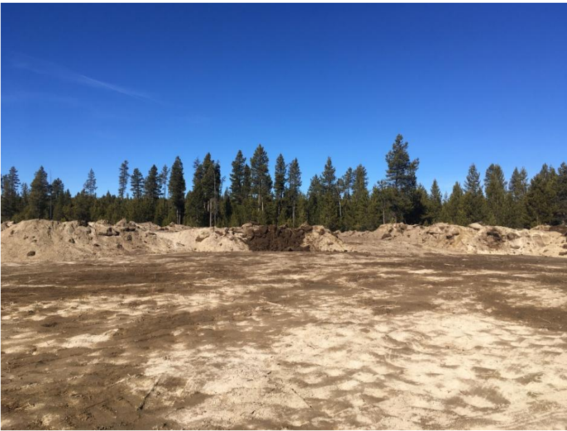
Figure 5: Looking West at the start of berm build-up along the western edge of the storage pond.
