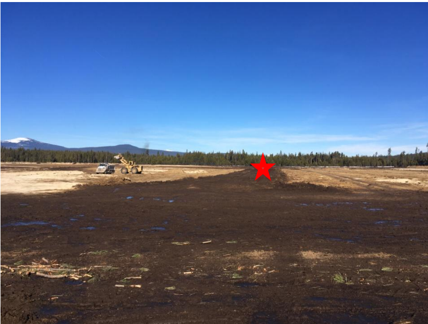
Figure 6: Looking North at the break between the two lagoons. This will be the future access to the Chlorination Building, with the star marking the approximate location of the Chlorination Building.
